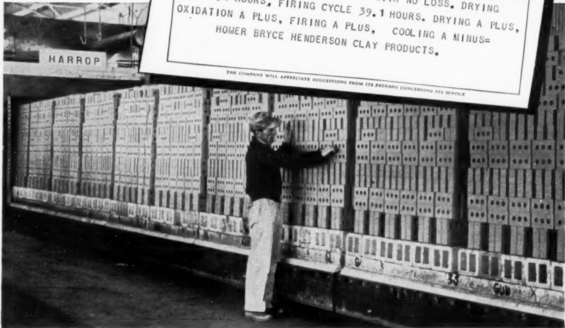
Latest Harrop Dryer and Kiln installation for Henderson Clay Products, Henderson, Texas. Twin Dryer is 184' long, Tunnel Kiln 421' long. Natural gas fired, with firing temperature approximately 2150°F.
